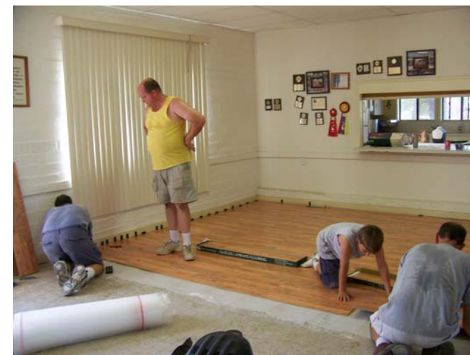
Tim Dunckel, Dave Fontana, Chris Dunckel and Chris Varvel laying down the new flooring.
